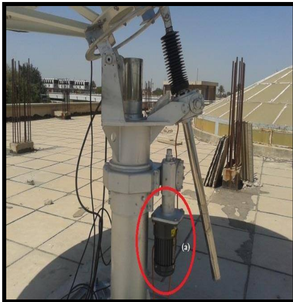
Figure 4. a- 3-Phase Az motor
